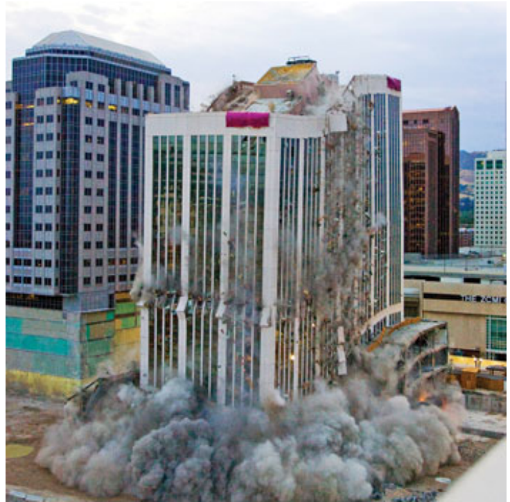
The 20-story Key Bank office tower was imploded, and replaced by the new 26-story Key Bank building, which sits in an active, multilevel pedestrian plaza, providing customers for the restaurants and cafés during the week. The project's below-grade parking structure was built on a large 30-by-60-foot (19.1 by 18.3 m) bay size not only to provide easily accessible parking with few columns, but also to permit the most flexibility in what was developed above. (William Tatham, SWA Group)
